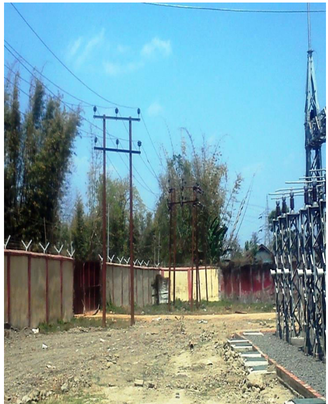
33 kV (H Pole) line inside substation
